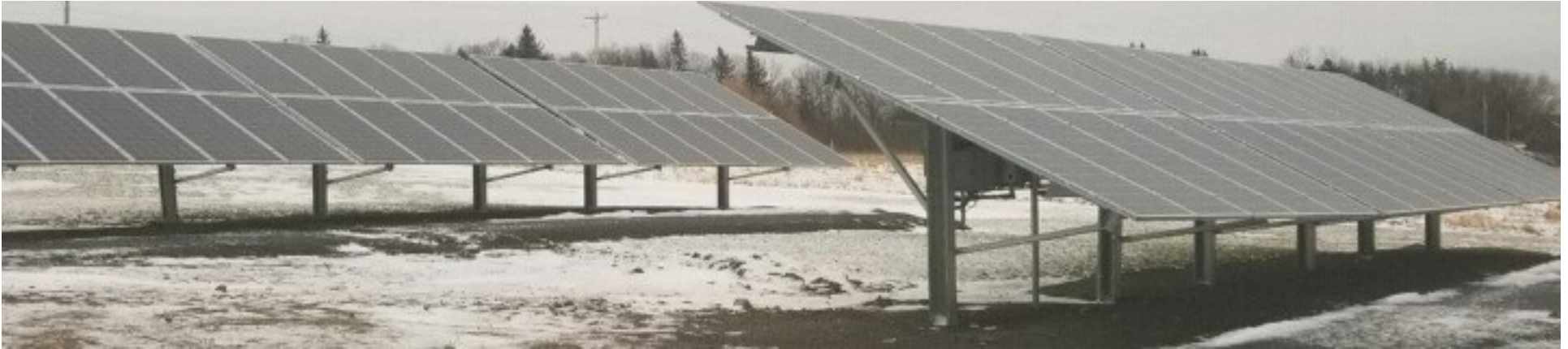
Town of Richland Solar Array; Photo Credit: CNY RPDB
